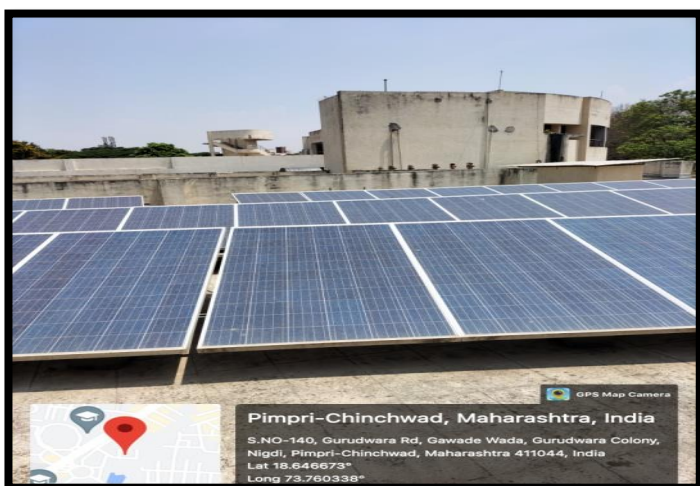
Roof Top Solar PV Plant
